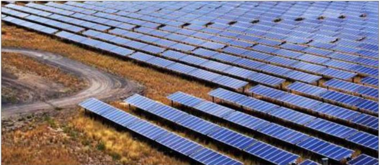
Figure 10 – Example of fully assembled tracking array
